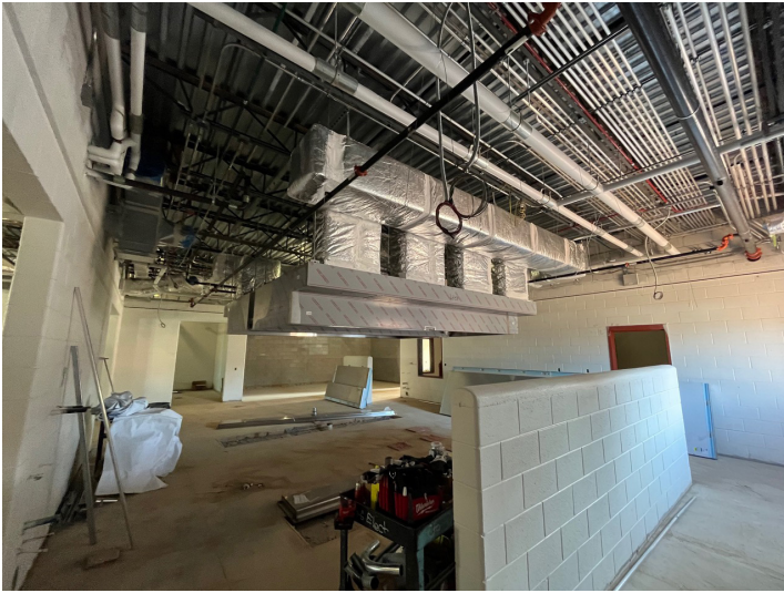
KITCHEN EXHAUST HOOD DUCTWORK
