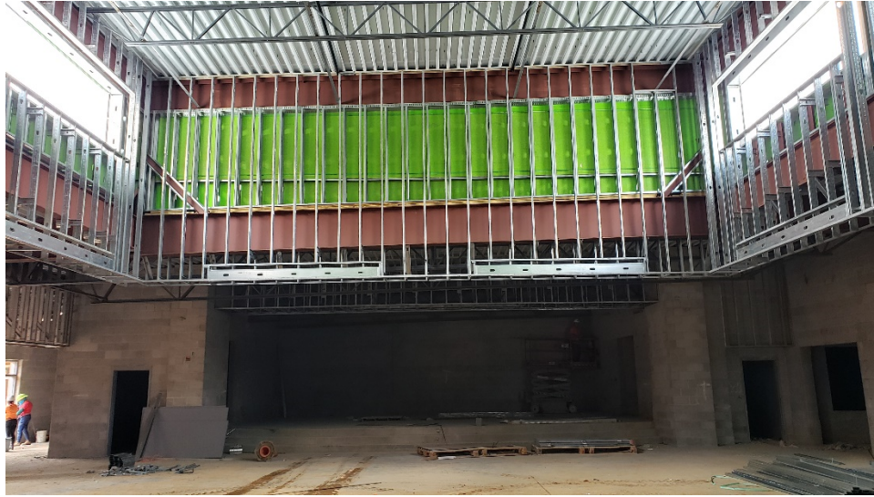
Area "C": Dining Area and Platform
