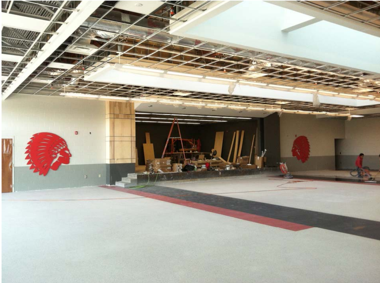
1 – Dining room interior. Clerestory windows in the roof monitors will allow natural light to illuminate the interior. Jackson Indians spirit graphics flank the stage. Floor is terrazzo, being final-polished in this photograph.
