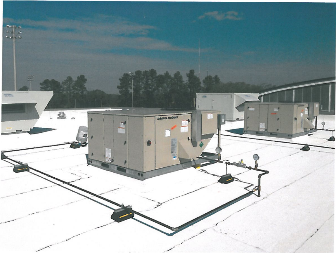
Field House Rooftop Units
